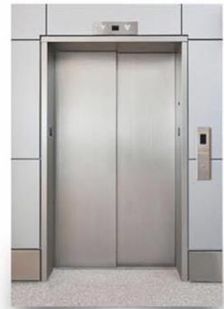
SS Center Auto Door Car & Landing
