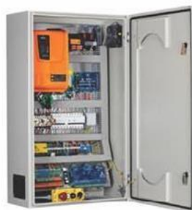
Integrated Control Panel
